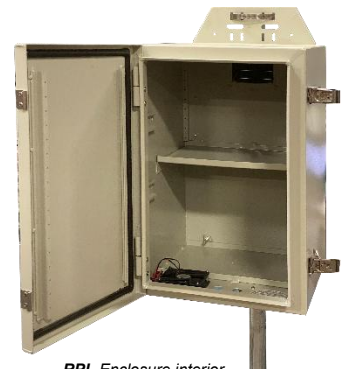
RPL Enclosure interior without batteries or controller
