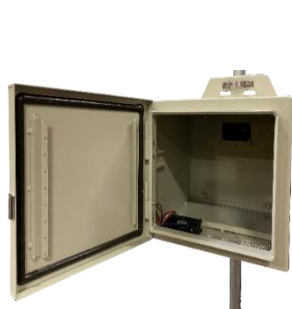
RPS Enclosure interior without batteries or controller
