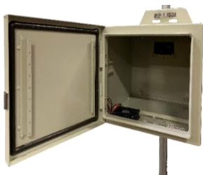
RPS Enclosure interior without batteries or controller
