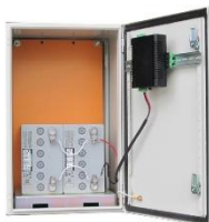
RPST with 100Ah of battery
