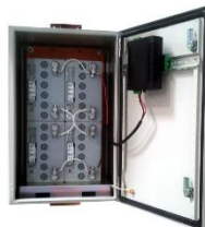
RPST with 200Ah of battery
